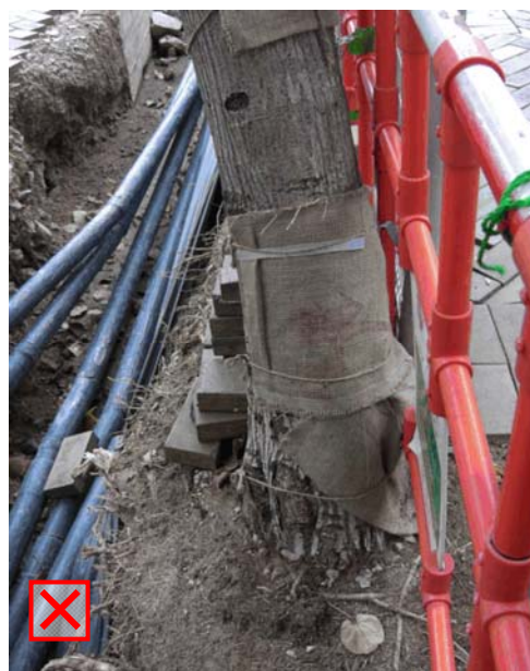
Photo 9 - Excavation within tree protection zone will cause significant damage to root system
