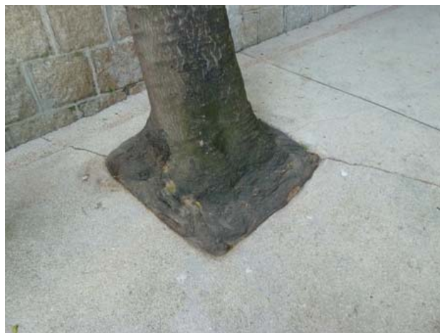
Fig. 6 A bad example showing a tree surrounded by concrete around the root collar
