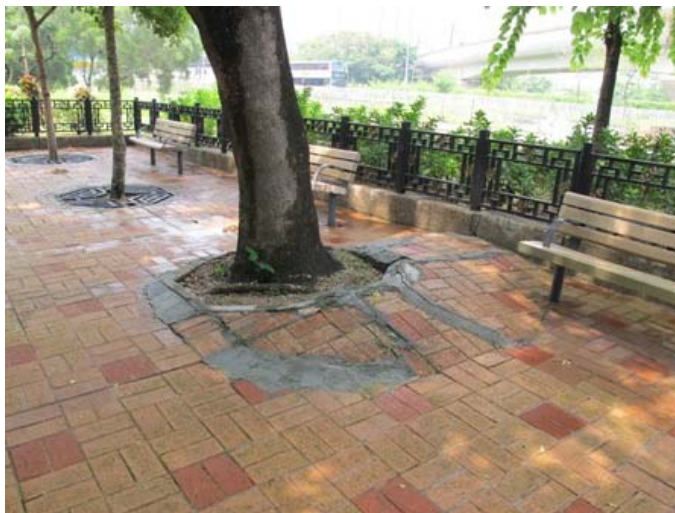
Fig. 2 Pavement lifting caused by root growth
