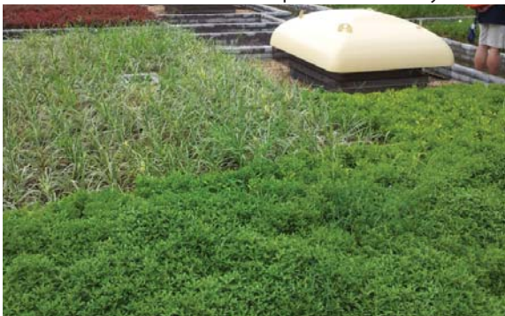
位於渠務署設施上的粗放型屋頂綠化 Extensive green roof at Drainage Services Department's facility
