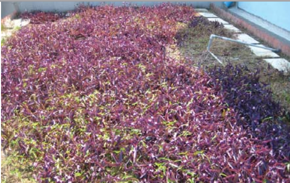
位於水務署設施上的粗放型屋頂綠化 Extensive green roof on top of the Water Services Department's facility
