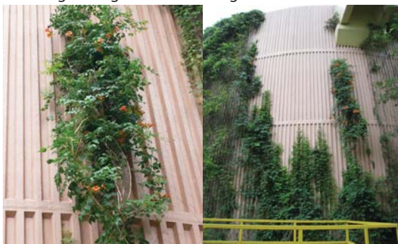
自行攀緣於沙田污水處理廠的外牆上 Self clinging on wall at Sha Tin Sewage Treatment Works
