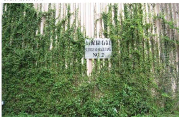
自行攀緣於沙田污水處理廠的外牆上 Self clinging on wall at Shatin Sewage Treatment Works
