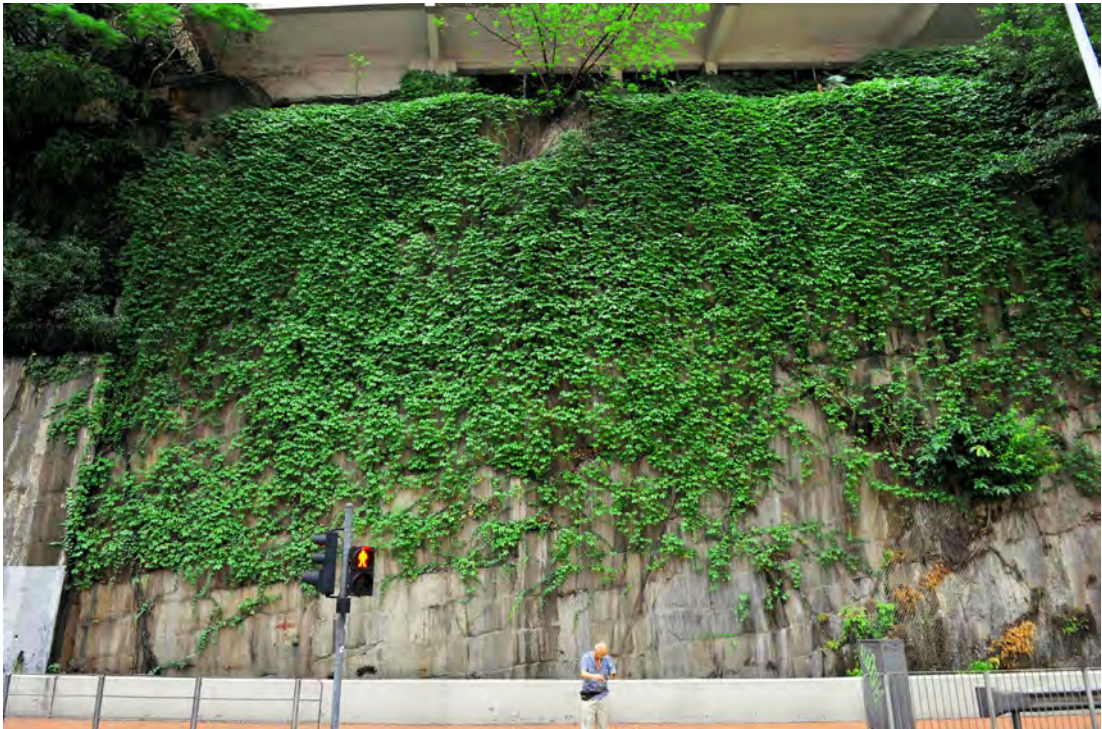
Wire mesh as a trellis for climbers to reduce the visual impact of a rock slope
