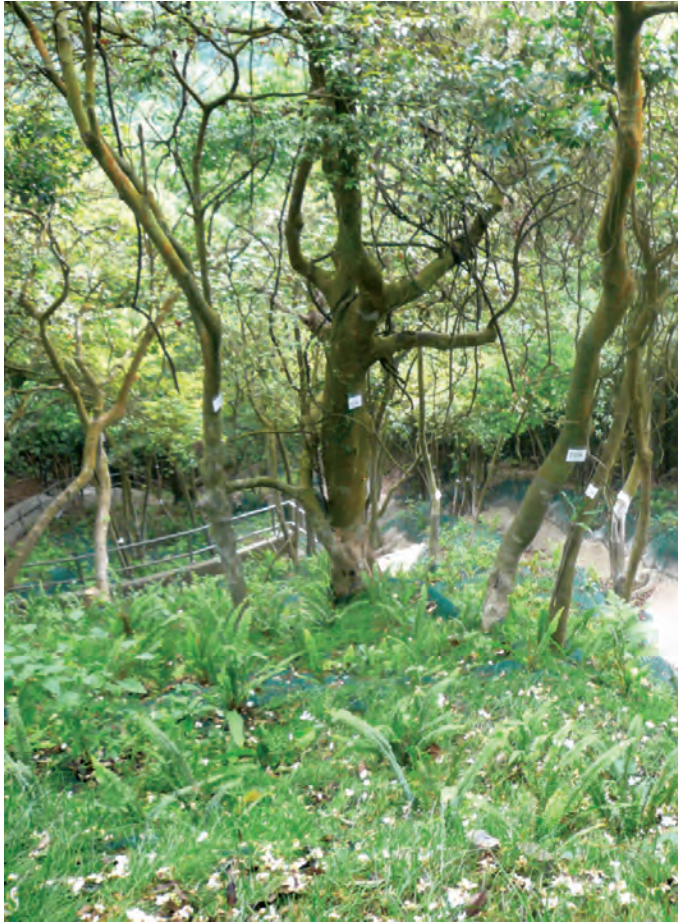
Ferns and other shade tolerant species under tree cover on a soil nailed fill slope
