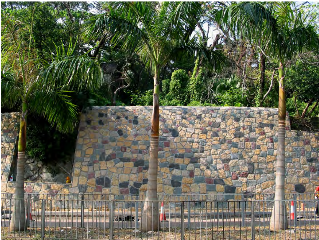
Coloured masonry facing to a skin wall (the pattern of masonry blocks followed the existing wall and the block size decreases with height)
