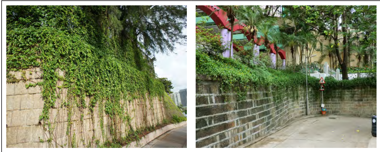
Figure 2.18 Trailing Plants Growing from the Crest of Retaining Walls
