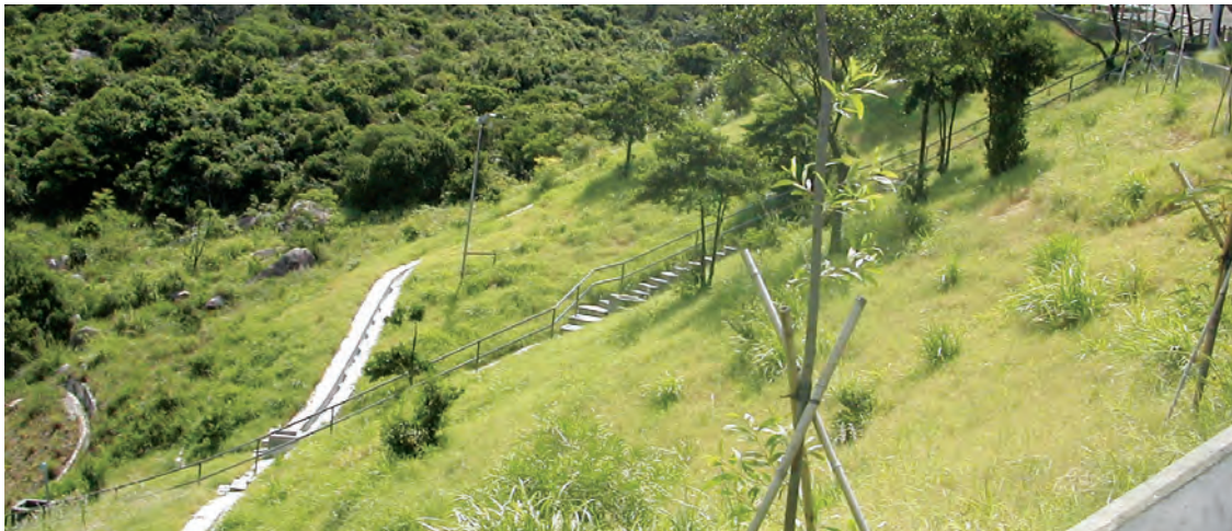
Grass and shrubs on a fill slope planted over a buried soil nail concrete grillage system
