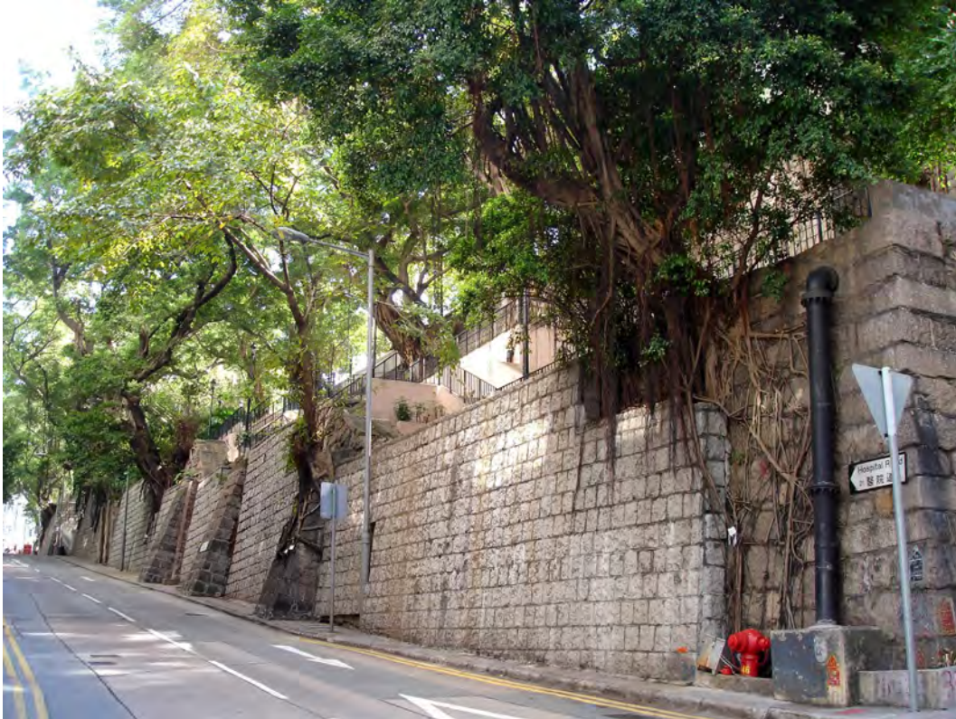
Preservation of wall trees on an old masonry wall with provision of skin wall with space left to accommodate the existing wall trees
