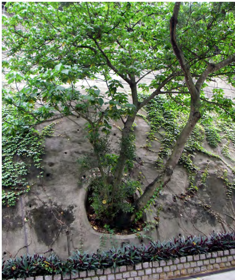
Provision of tree rings to retain existing trees and use of limited available space for planters (planting climbers to reduce visual impact of a hard surface)
