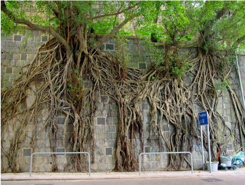
Soil nail heads located beneath granite finish textured blocks on an old masonry wall with existing wall trees
