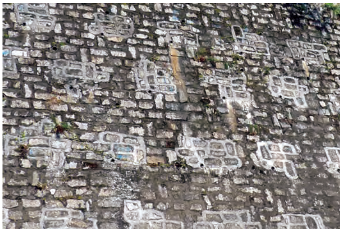
(b) Unsatisfactory appearance of soil nails heads beneath stone pitching
