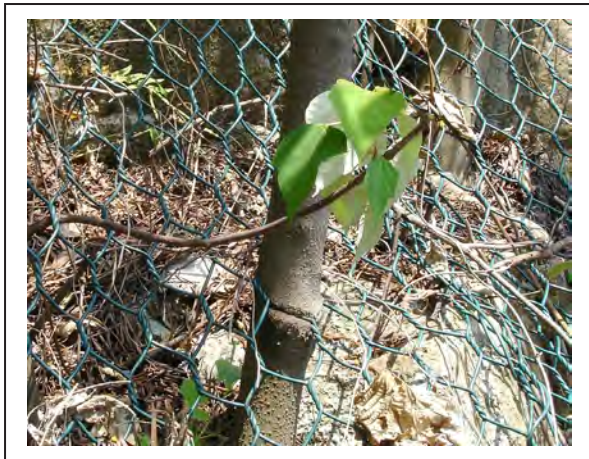
Figure 2.20 Unsatisfactory Interaction of Wire Mesh and Vegetation
