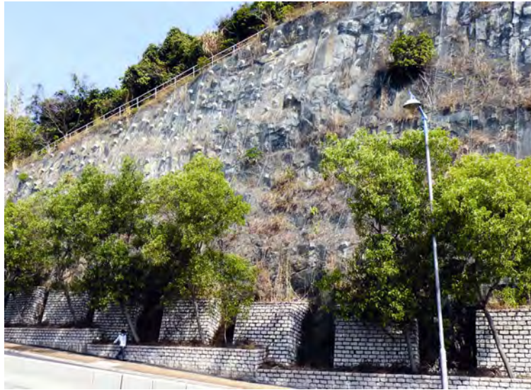
Masonry facing to buttresses and toe planter for rock slope (screen planting further softens the appearance of visually sensitive area at the lower portion of the slope)
