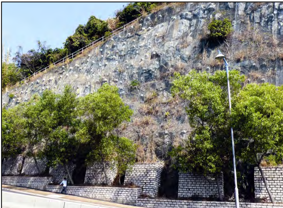
Recent photograph of slope appearance (2011)
