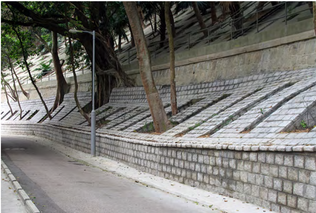
Openings in a soil nailed fill slope using grillage system to retain the existing trees (grillage covered in masonry facing)
