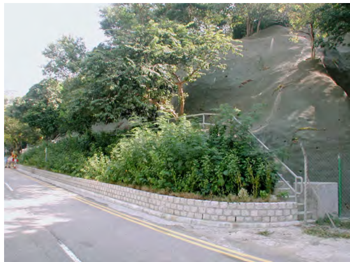
Masonry planter wall, coloured handrails and sprayed concrete hard surface to upper slope
