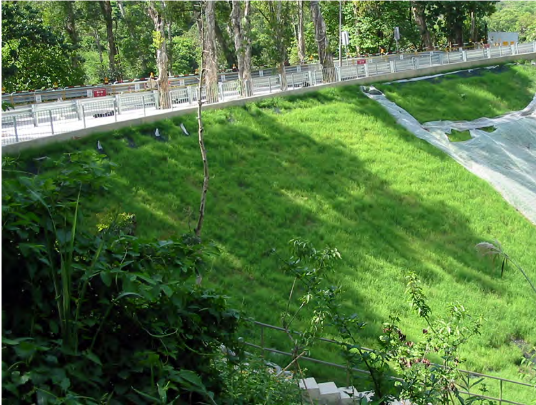
Well established hydroseeded grass on a rockfill slope with soil cement mix overlay
