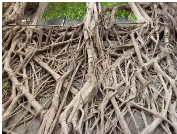
Photo No. 1 – Distinctive root network on retaining wall surface
