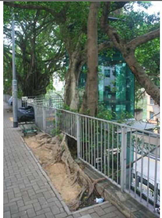
Photo No. 7 – Provision of rooting areas at the crest of the retaining wall
