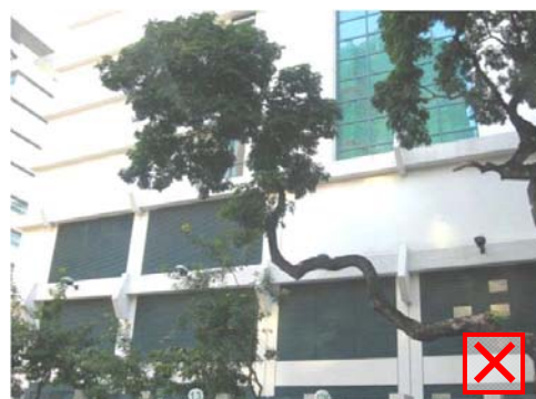
Photo 5 - Improper pruning caused by excessive removal on inner branches results in over lifting of crowns and lion-tailing.
