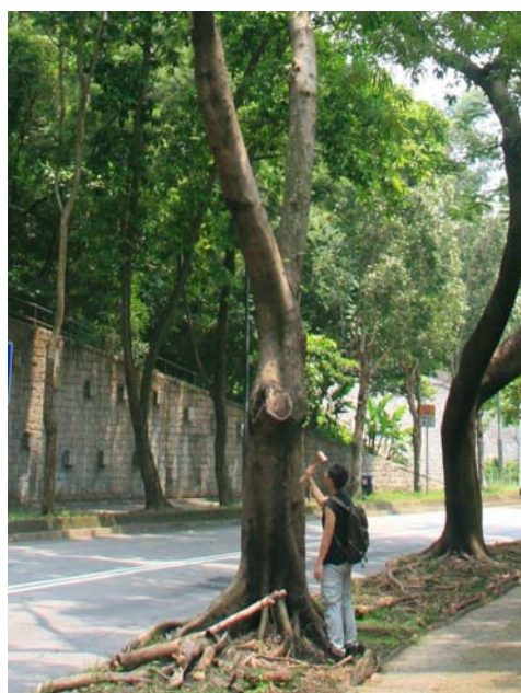
Photo 1 - Conduct sounding test by a mallet to assist in estimating the presence of internal decay
