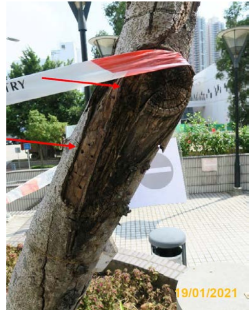
Pest(borer) and Decay
