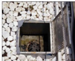
Inspection Chamber for Rain Outlet Protection
