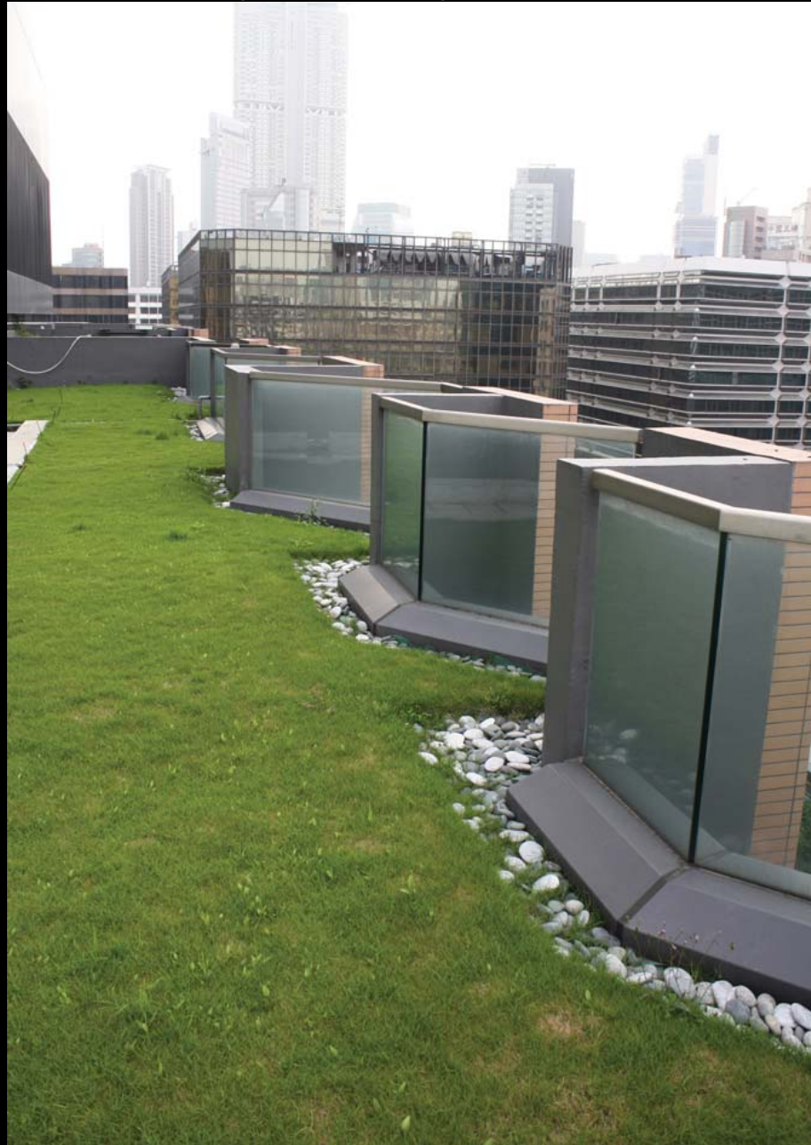
Green roof at top roof of staff quarter 員工宿舍綠化屋頂
