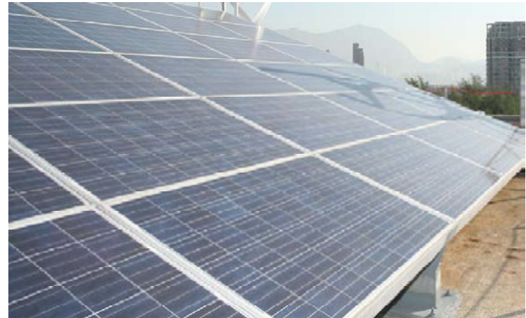
Photovoltaic (Solar) Panels
