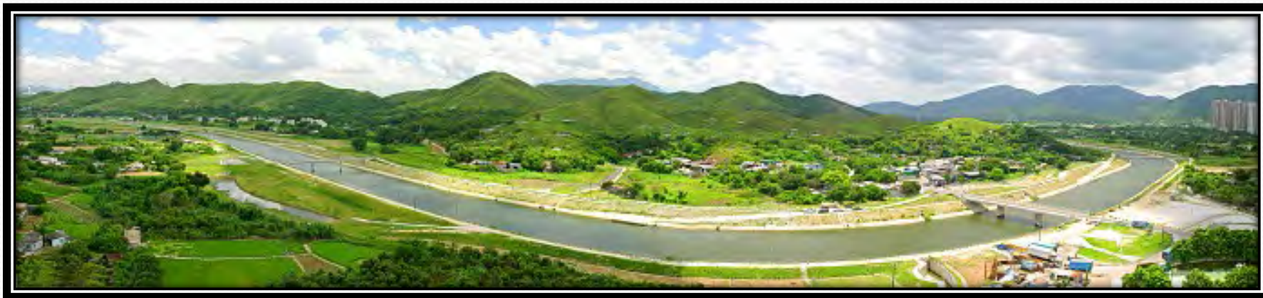
Completed river training works at Ng Tung River near Tin Ping Shan, Sheung Shui
