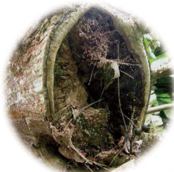
Wood decay / cavity 腐壞 / 樹洞
